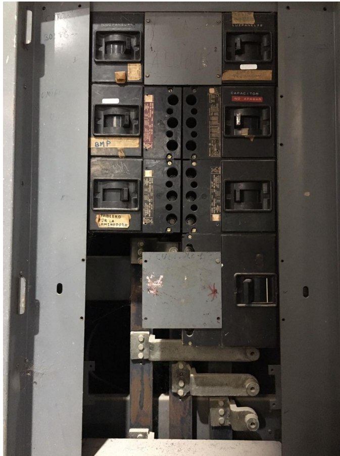
Figura 3.19 Tablero principal acometida 2
