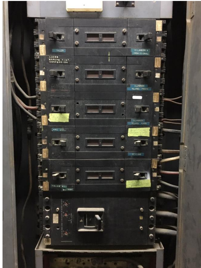
Figura 3.18 Tablero principal acometida 1
