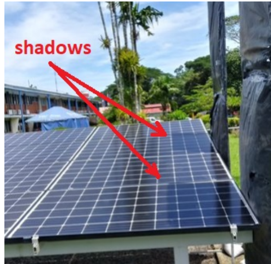
Fig. 9. Example of partial shadows generated on the PV modules.
