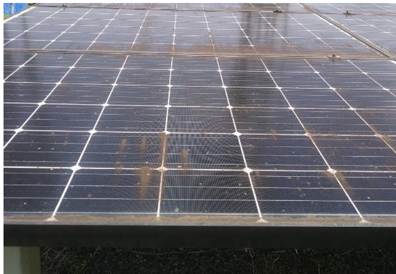
Fig. 3. Monocrystalline PV module used in this research for the evaluation of natural soiling. It is possible to observe the presence of non-uniform dirt.
