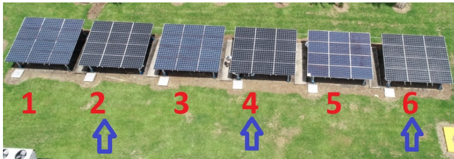
Fig. 3. Picture of the PV installation. Strings 2, 4 and 6 were used in this research.
