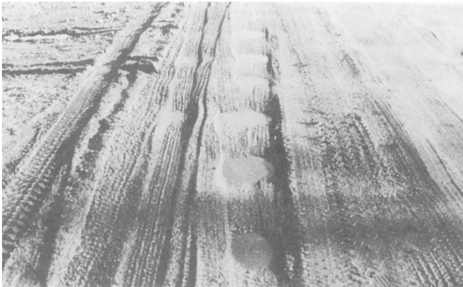
Figure B-6. Medium severity example of corrugations.
