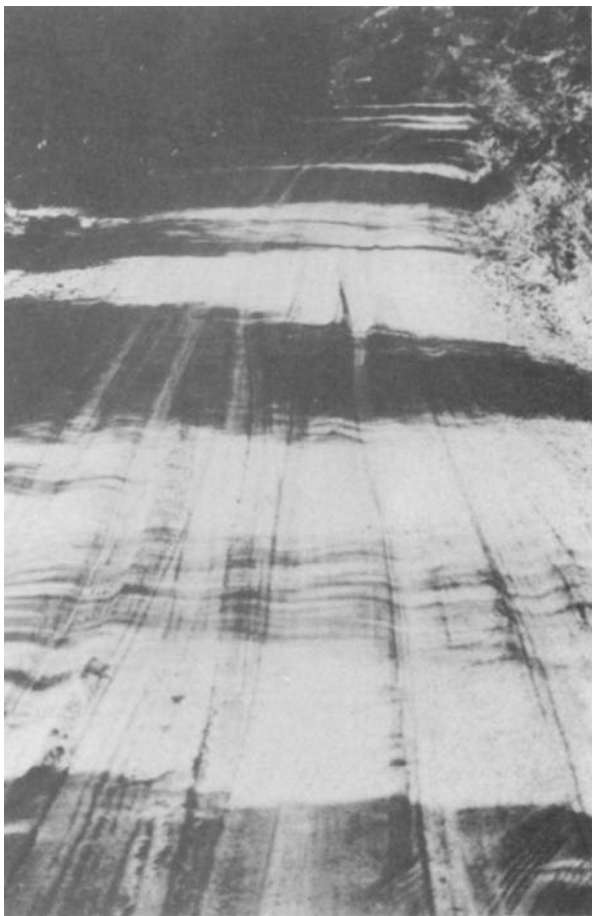
Figure B-12. Low severity example of ruts.
