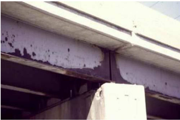
Figure 1. Typical location of corrosion in steel beam.
