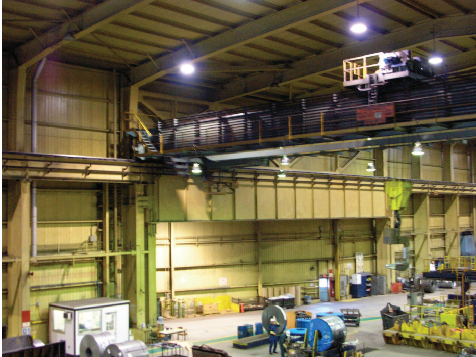
Photo 3 – 50 Ton Coil Handling Crane
