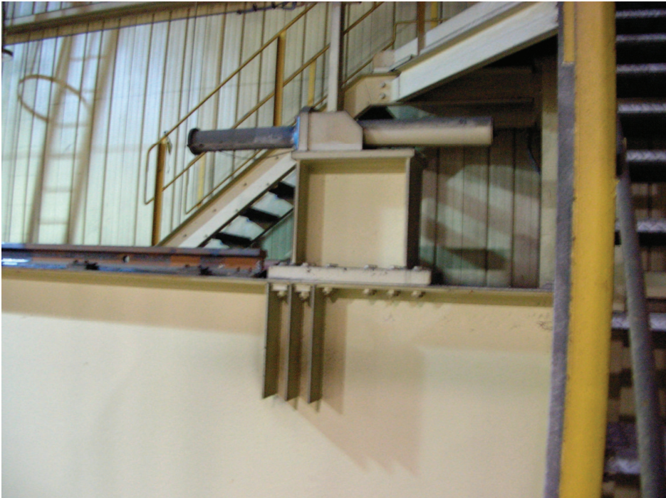
Photo 2 – Crane Runway Bumper Stop with Hydraulic Bumper
