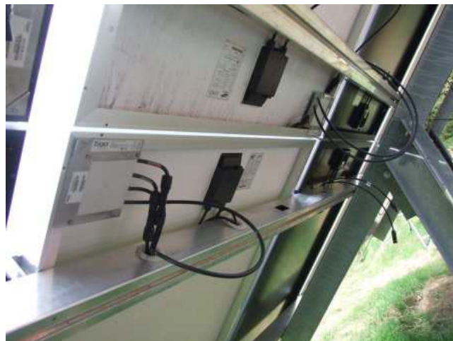
Figura 8-9 Optimizer conectado a un panel, PV Test Station
